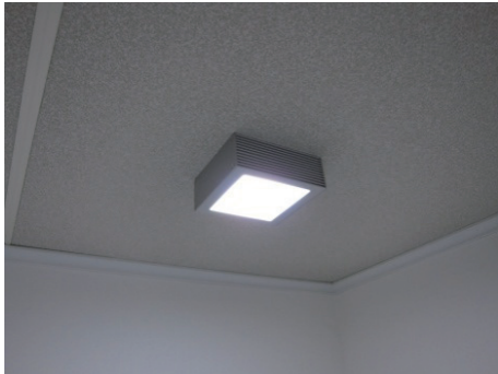
Special LED light (with controller unit)
